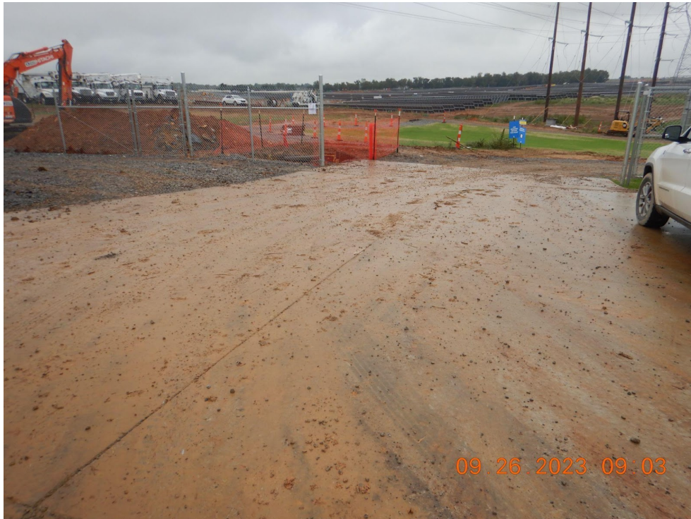
Inadequate construction entrance installed to prevent track out from the site.
