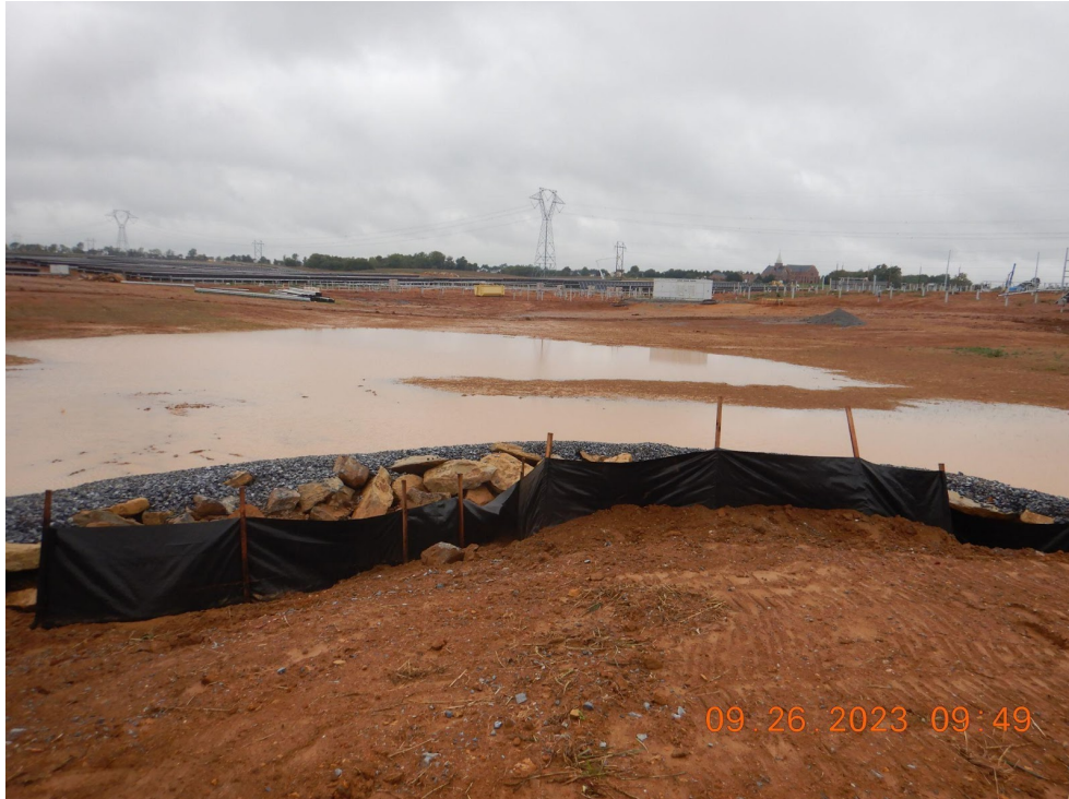
Sediment Pond 14 has been converted to final stormwater management pond prior to all uphill disturbance being vegetated.
