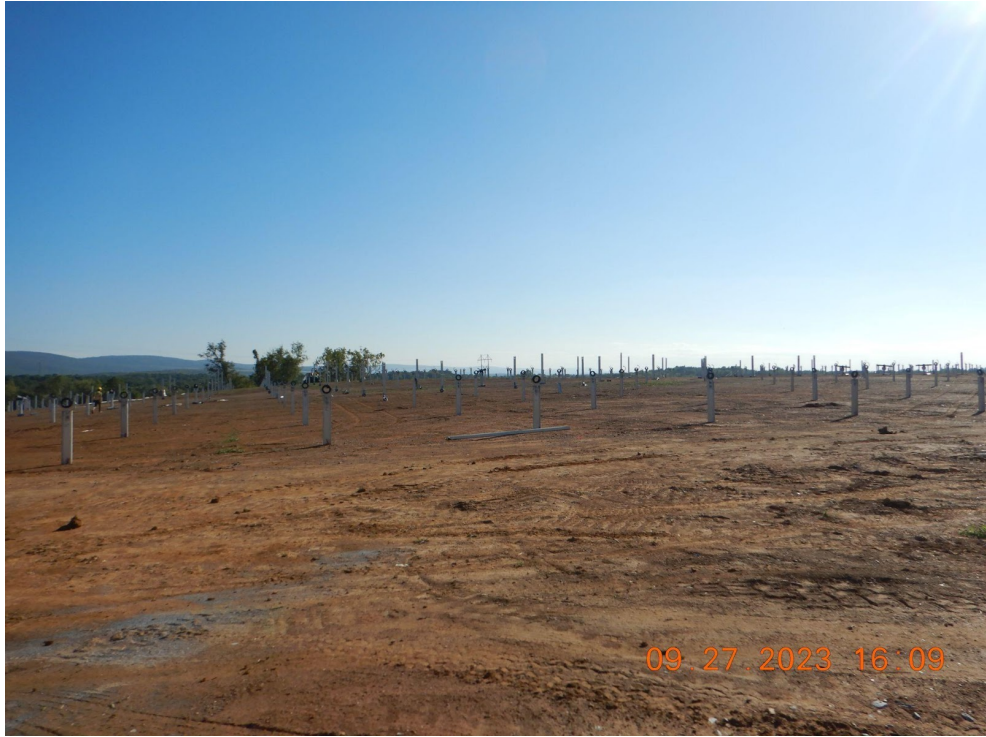
Unstabilized area of project. Temporary or permanent stabilization hasn't been started.
