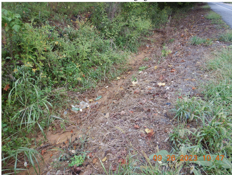
Sediment laden water across road from sediment basin 6 into an Ephemeral UNT of Evitts Run (39° 15' 33.3189" X -77° 49' 30.6042").
