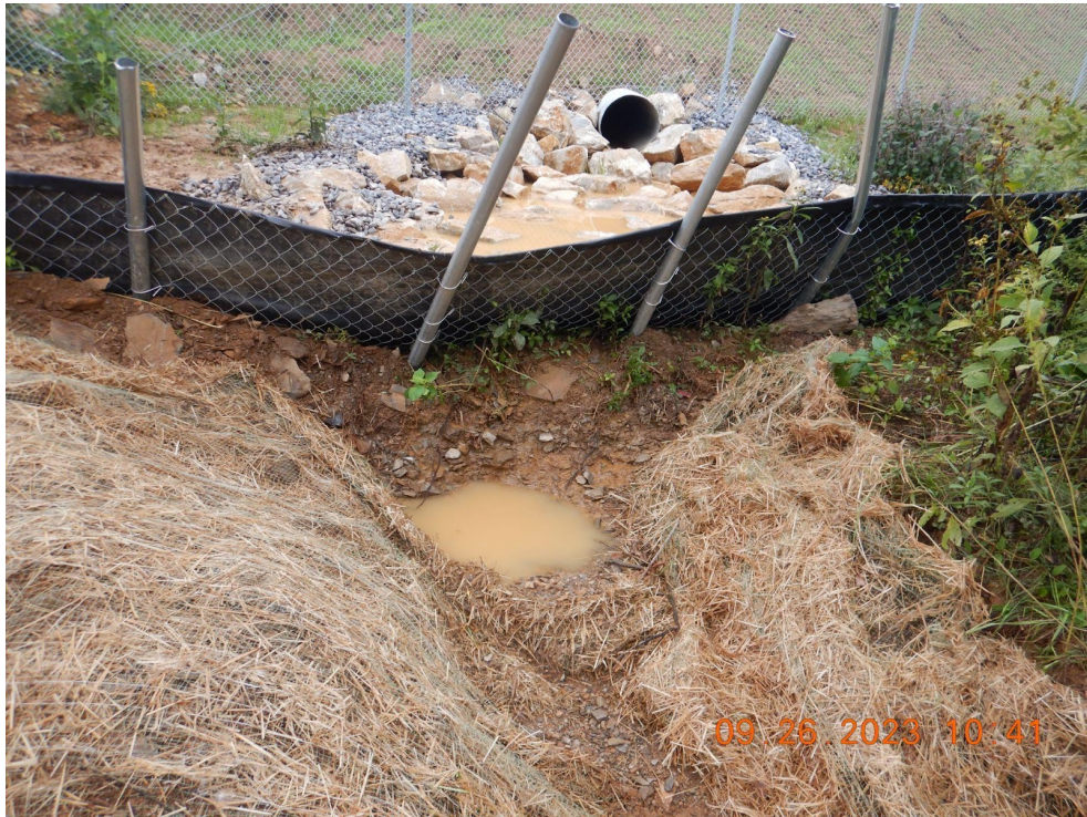
Area of Sediment Basin 6. Sediment Laden water leaving site through outlet. No outlet sign is visible.
