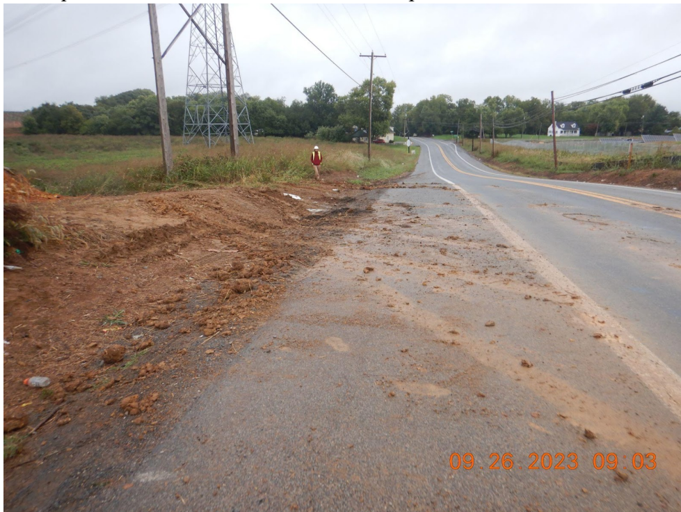
Unstabilized construction entrance.
