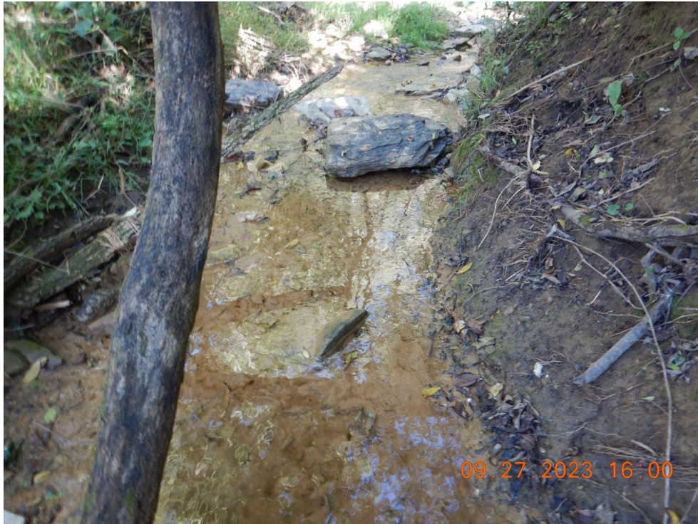
Sediment deposits into onsite UNT Evitts Run from Sediment Basin 5.
