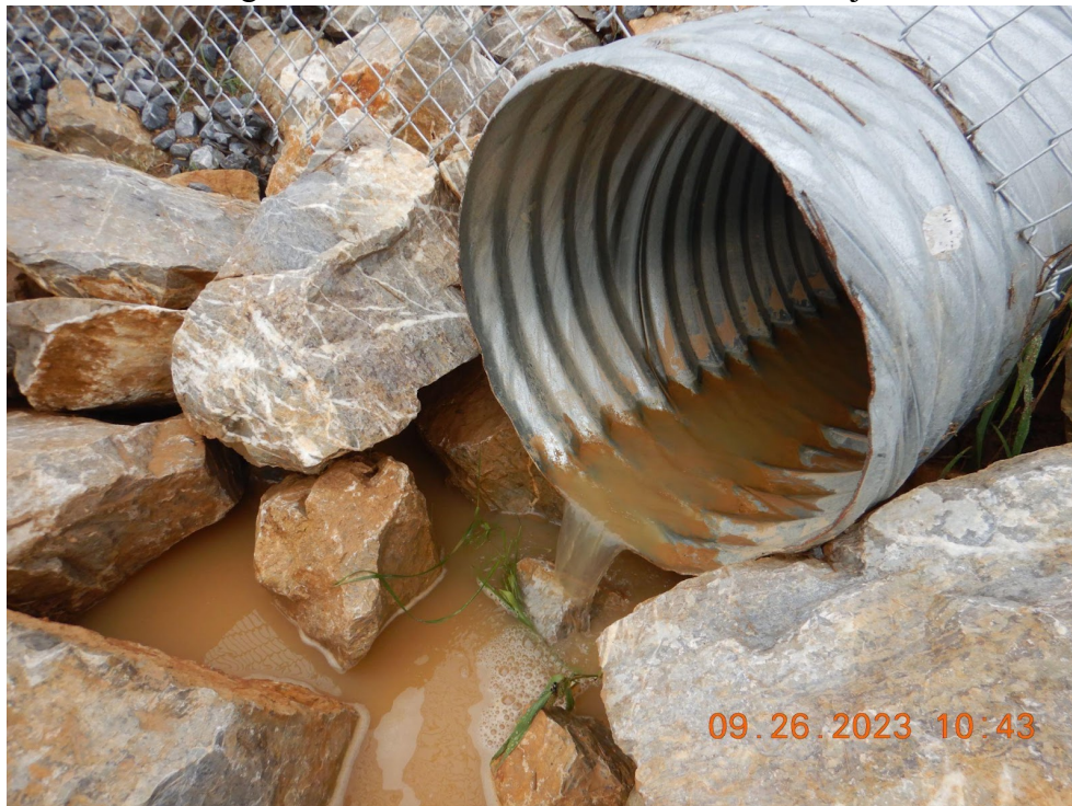
Sediment laden water discharging from Basin 6.
