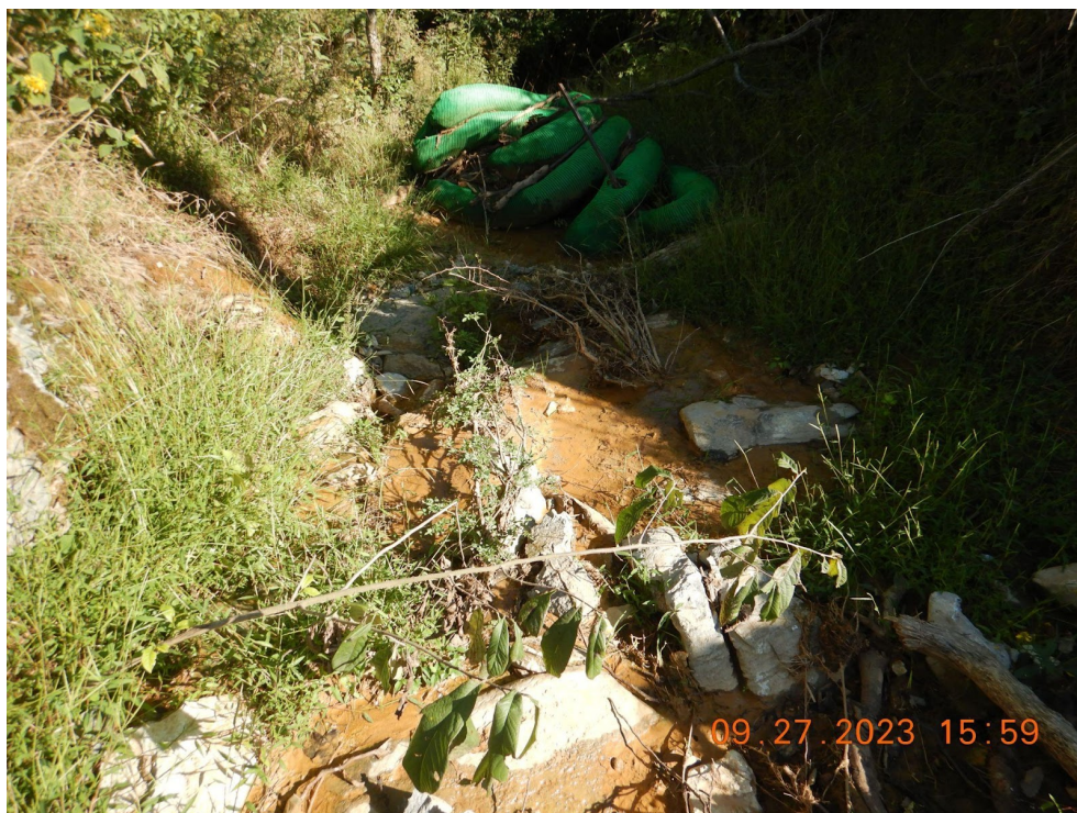
Sediment laden discharge from sediment basin 5 into onsite UNT Evitts Run.
