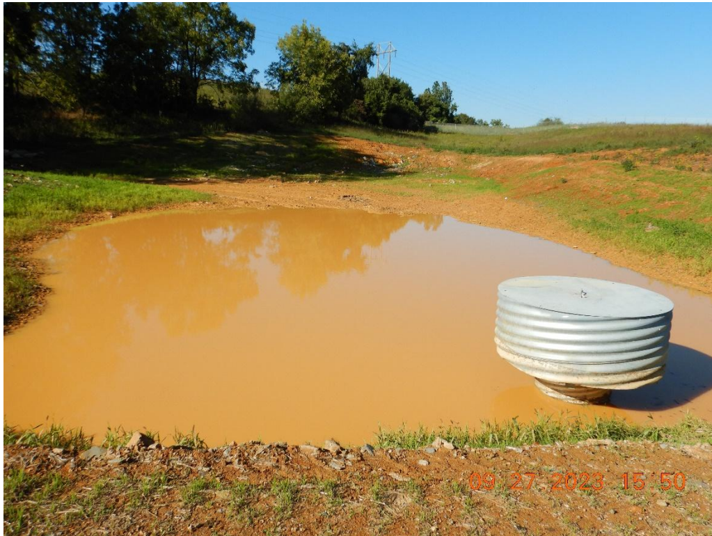
Sediment Pond 5 showing the lack of a stabilized inlet.
