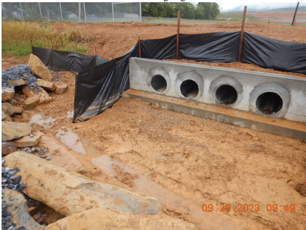
Outlet for stormwater pond 14 has been installed. Sediment laden water leaving site through outlet.
