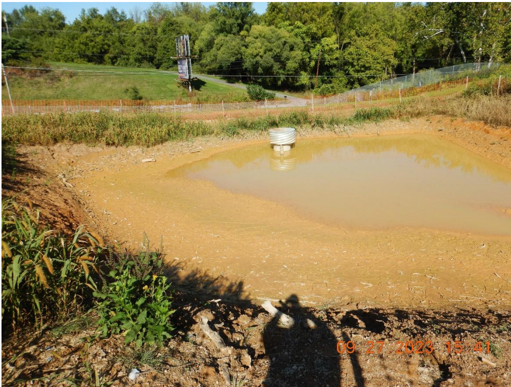
Sediment basin 6 showing the amount of accumulated deposits.
