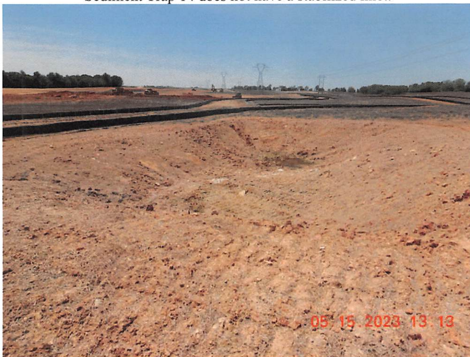
Sediment Trap 16 has no stabilized inlet or outlet.
