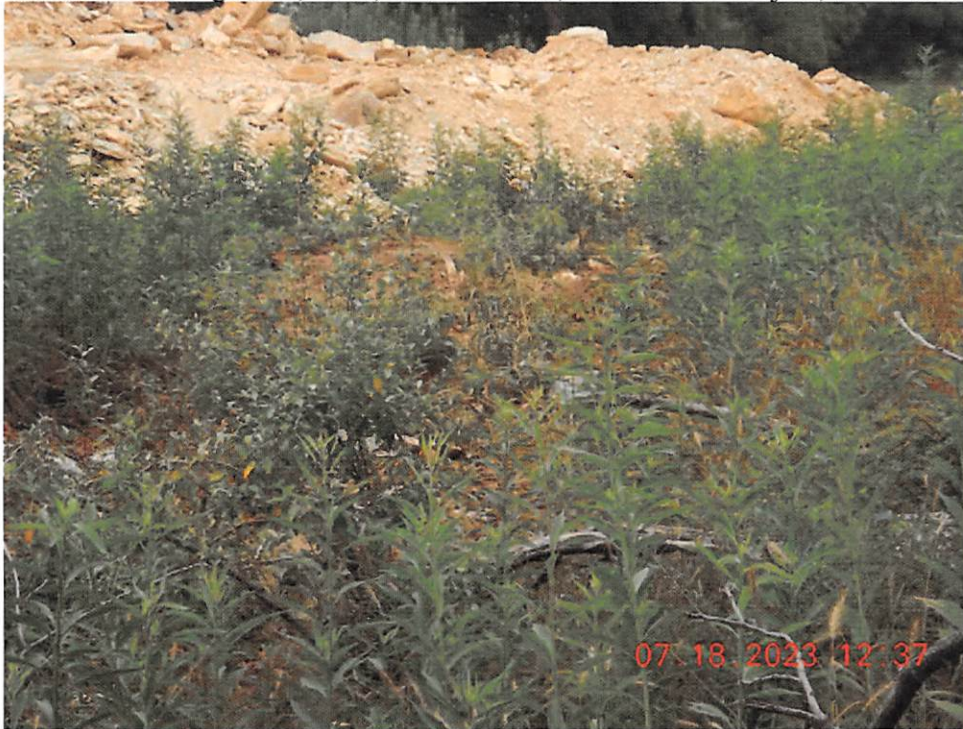
Area where Sediment Basin 5 should be installed and is not.
