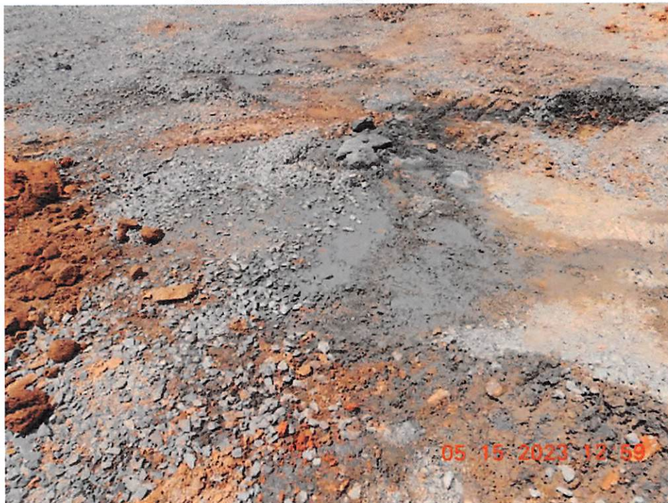
Concrete washout is not being used properly.
