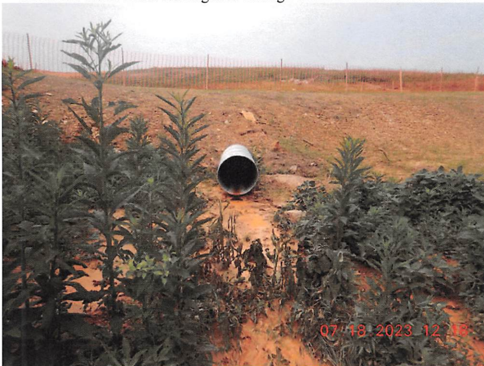
Outlet of Sediment Basin 6. No marker/sign for outlet.
