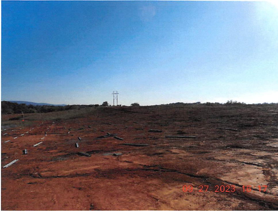
Unstabilized area of project. Temporary or permanent stabilization has not been started.
