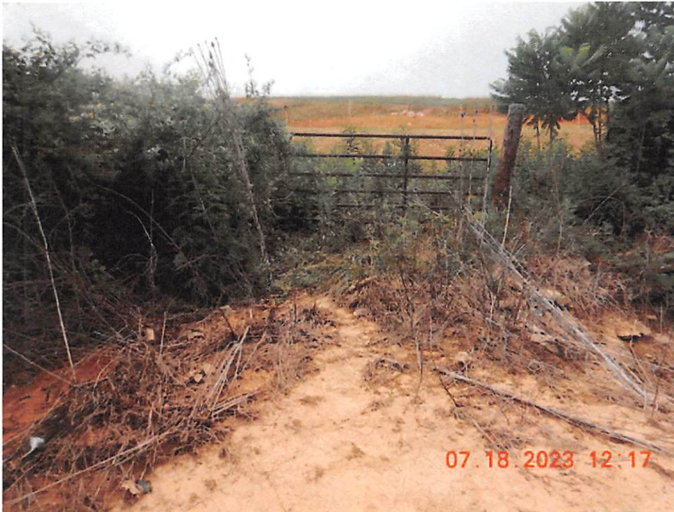
Sediment laden water leaving area through outlet of Sediment Basin 6.
