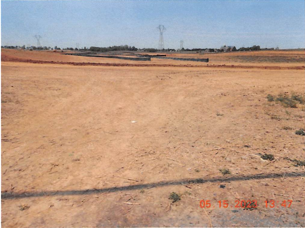
Construction entrance needs stabilization.
