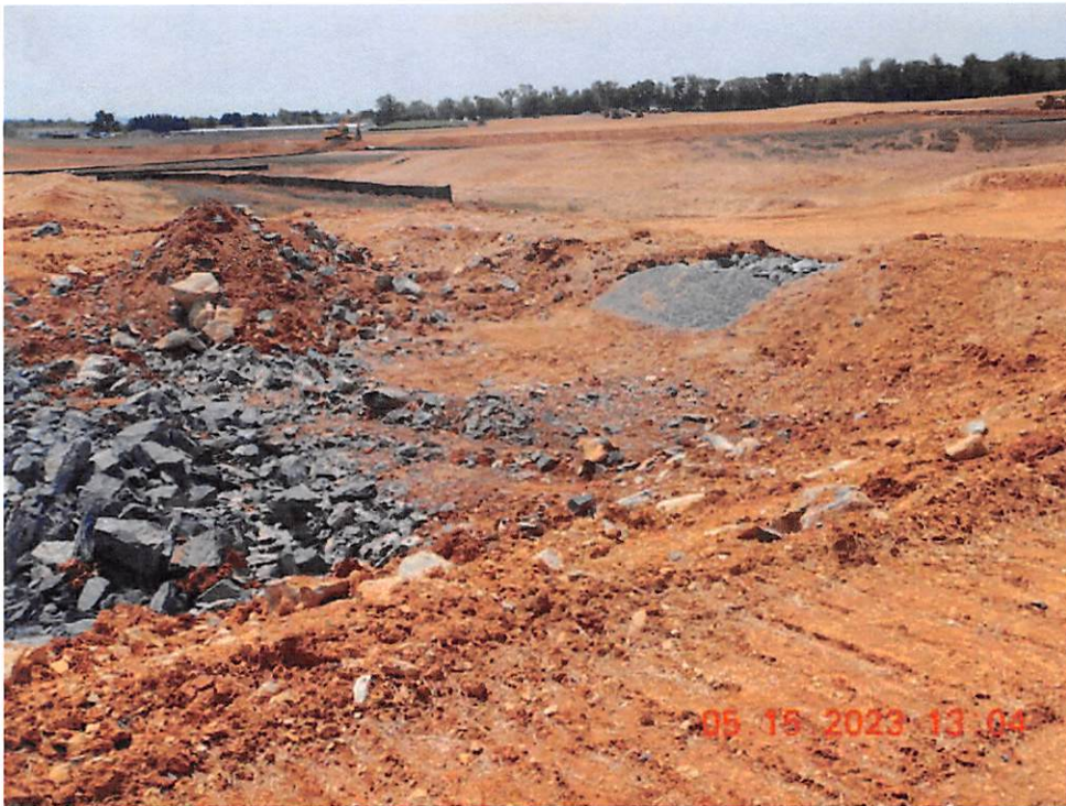
Sediment Trap 11 has no inlet, outlet marker, or Super Silt fence.
