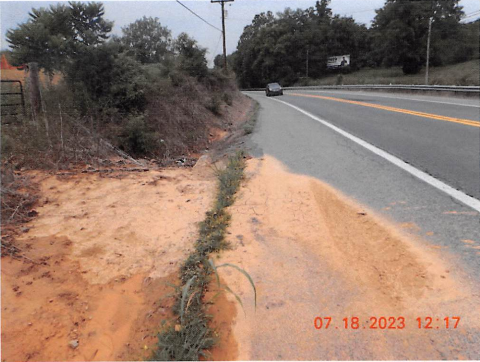
Outlet drainage area of Sediment Basin 6, discharging into WVDOH right of way
