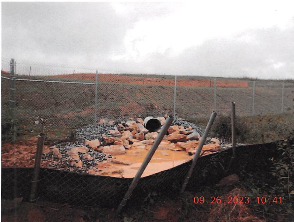
Sediment laden water leaving Sediment Basin 6. No outlet sign is visible.
