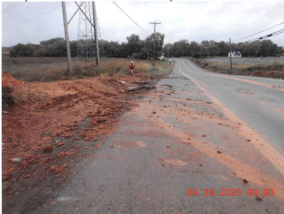
Unstabilized construction entrance.
