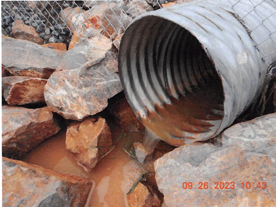
Sediment laden water discharging from Sediment Basin 6.
