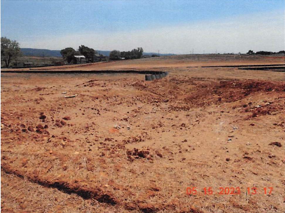
Sediment Trap 10 has no stabilized Inlet or Outlet.
