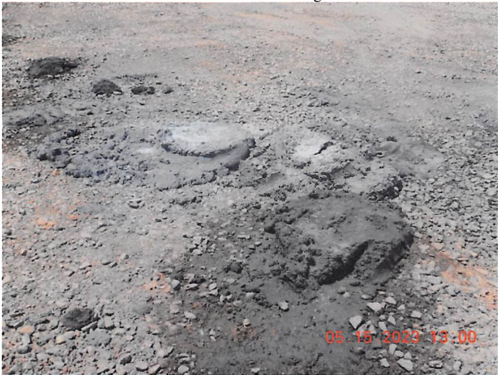
Concrete washout not being used.
