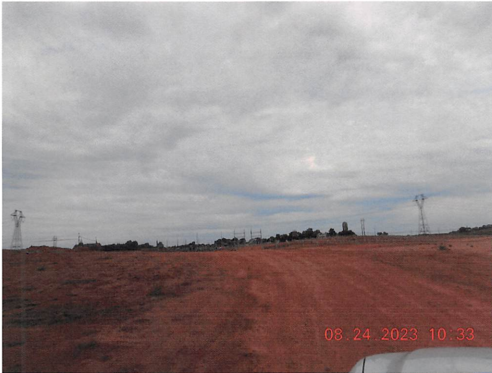
Area that has not been worked within the past 14 days and lacks temporary stabilization.
