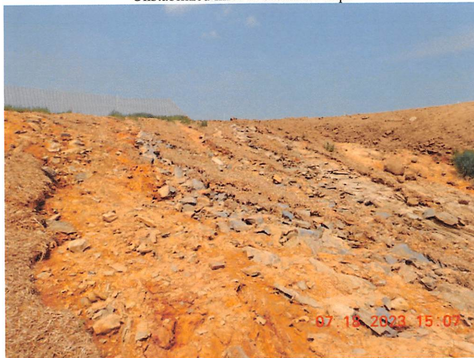
Erosion rills need stabilization.
