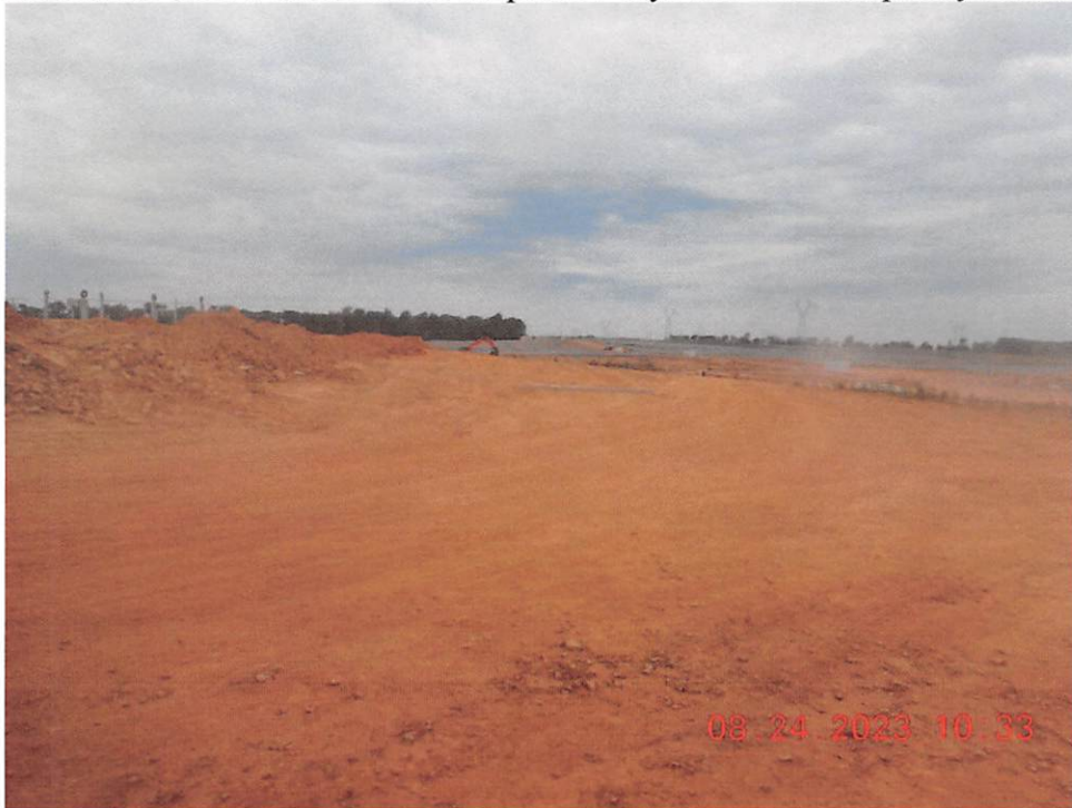
Area lacks temporary stabilization.
