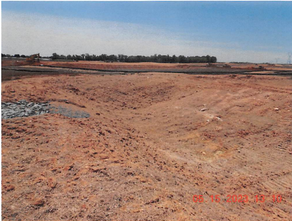
Sediment Trap 14 does not have a stabilized inlet.
