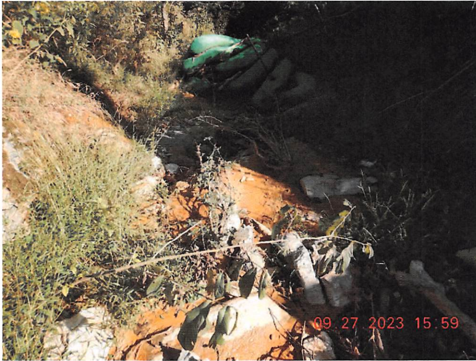
Sediment laden water discharged from Sediment Basin 5 into the UNT of Evitts Run.
