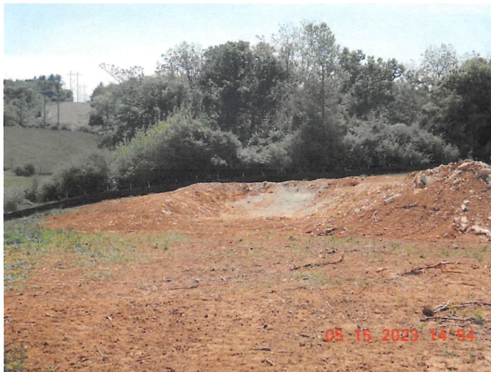
Sediment Trap 6 not finished. No stabilized Inlet or Outlet.
