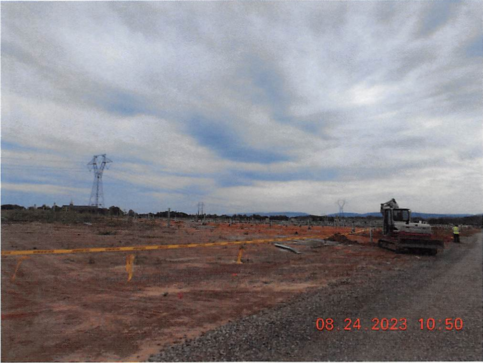
Area that lacks stabilization.
