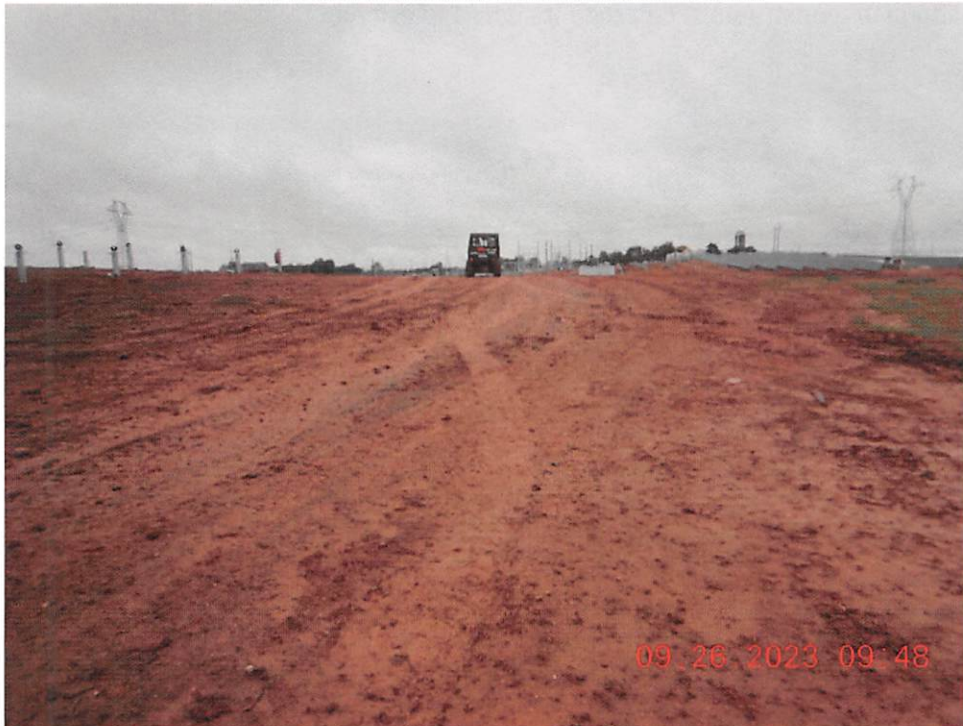
Unstabilized area of project. Temporary or permanent stabilization has not been started.
