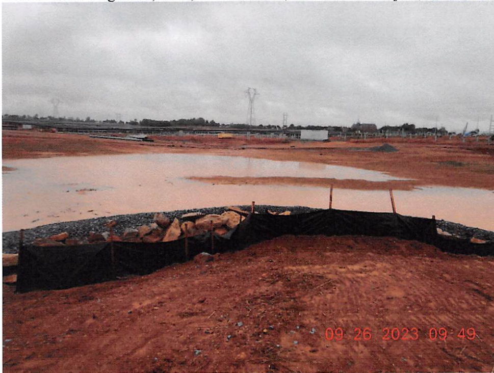
Sediment Pond 14 has been converted to a final stormwater management pond prior to all uphill disturbance being vegetated.
