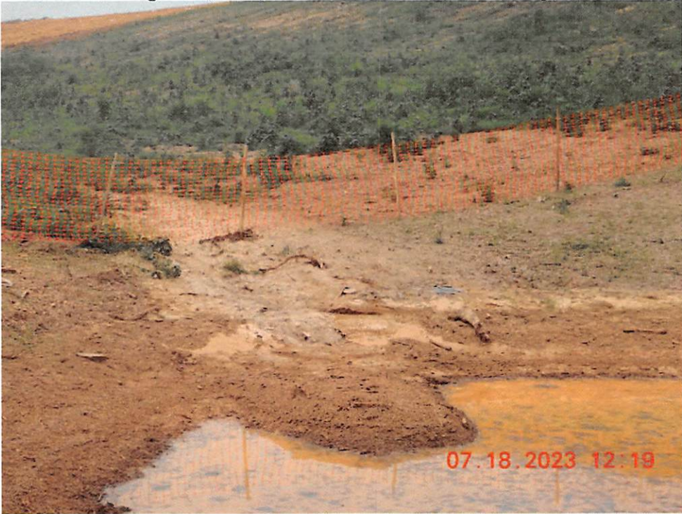
Unstable inlet to Sediment Basin 6.
