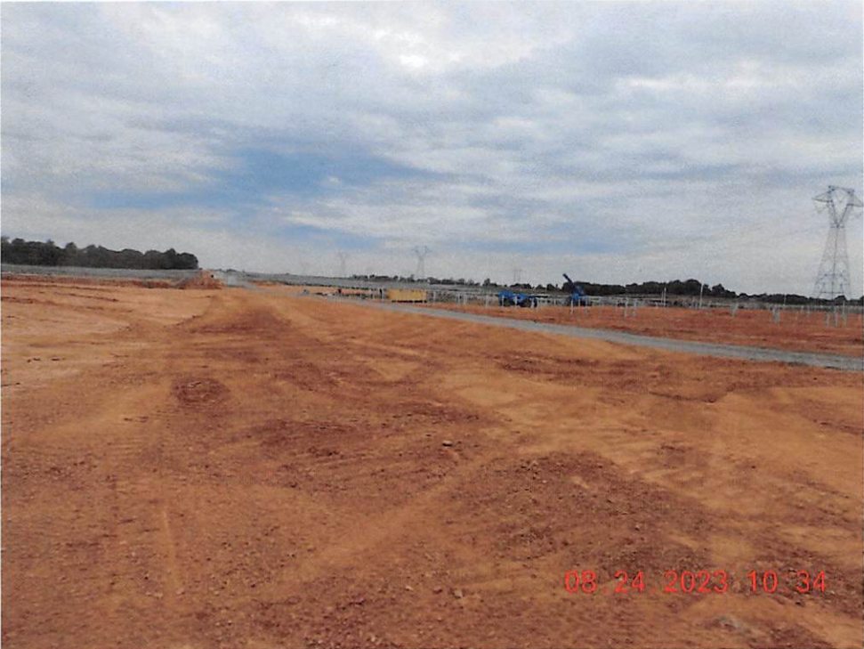
Area that lacks stabilization.
