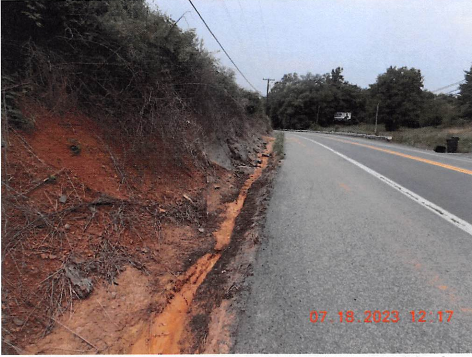
Sediment laden water leaving the project area through WVDOH right of way.
