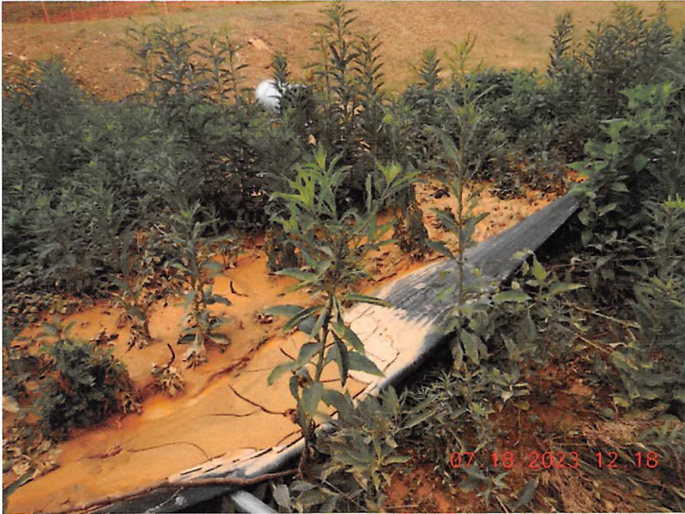
Super Silt fencing at lower end of outlet of Sediment Basin 6 needs maintenance
