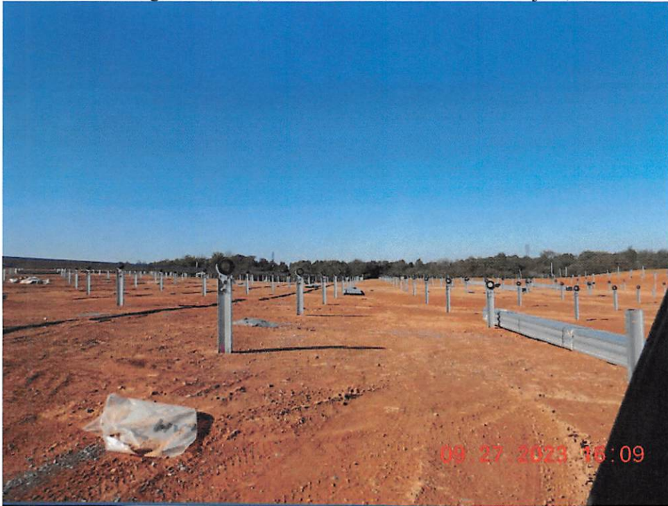
Unstabilized area of project. Temporary or permanent stabilization has not been started.
