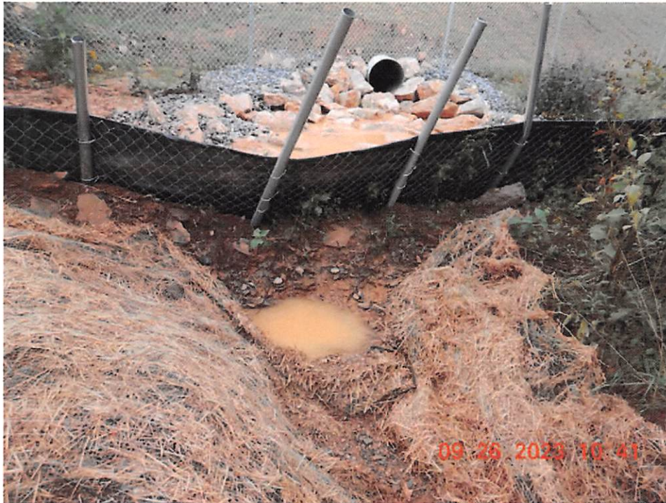
Area of Sediment Basin 6. Sediment laden water leaving site through outlet. No outlet sign is visible.
