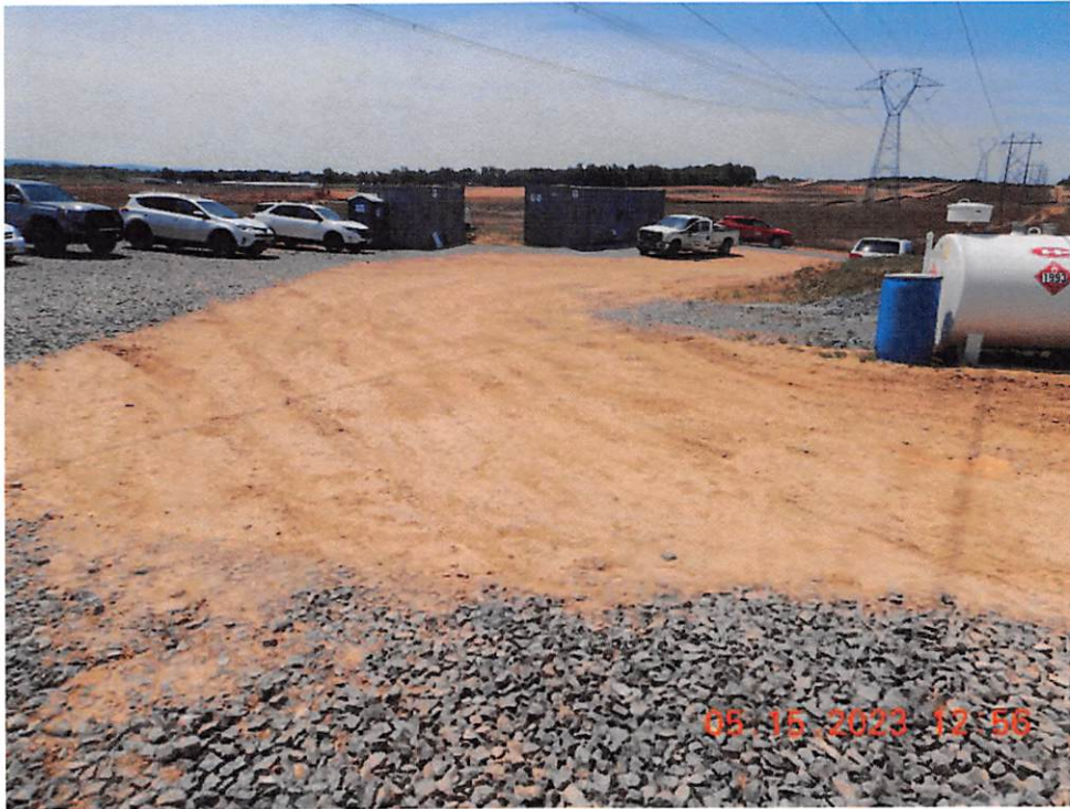
Unstabilized construction entrance.
