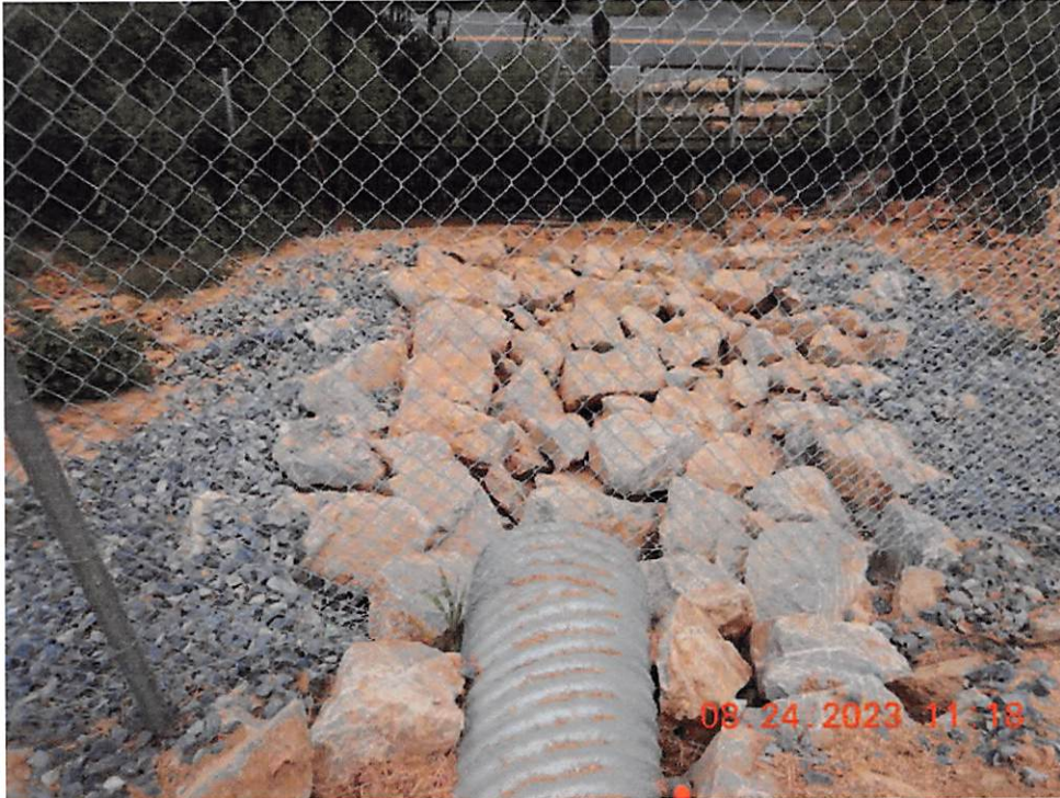
Area of Sediment Basin 6. No outlet marker has been installed.
