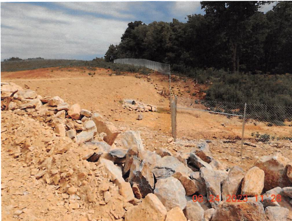
Area of Sediment Basin 5. Lacks stabilization and outlet marker.
