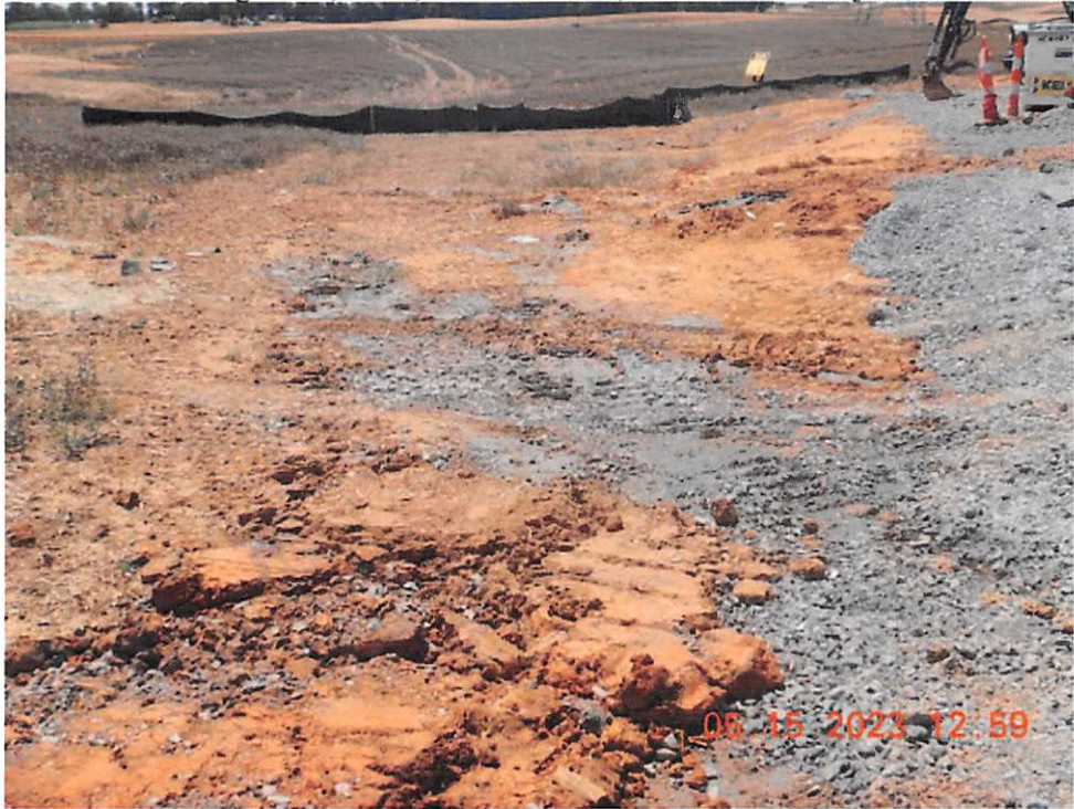
Concrete washout not being used.
