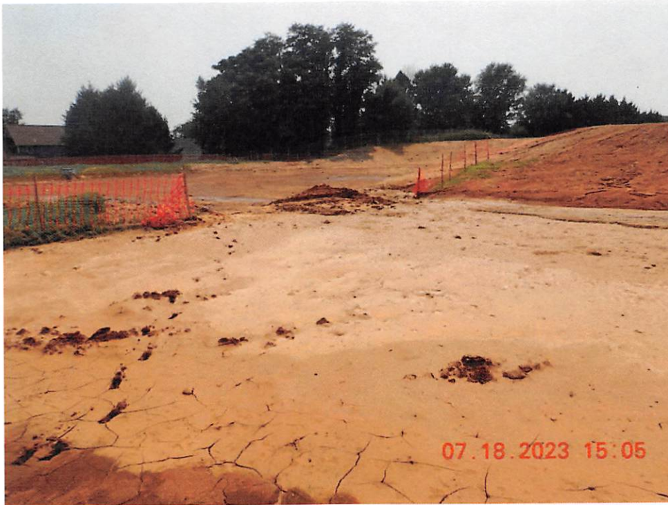
Unstabilized inlet of sediment trap.
