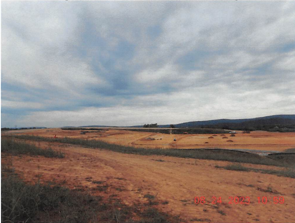
Area that lacks stabilization.
